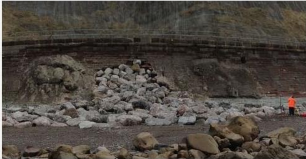
Hole in sea wall filled with rock armour
