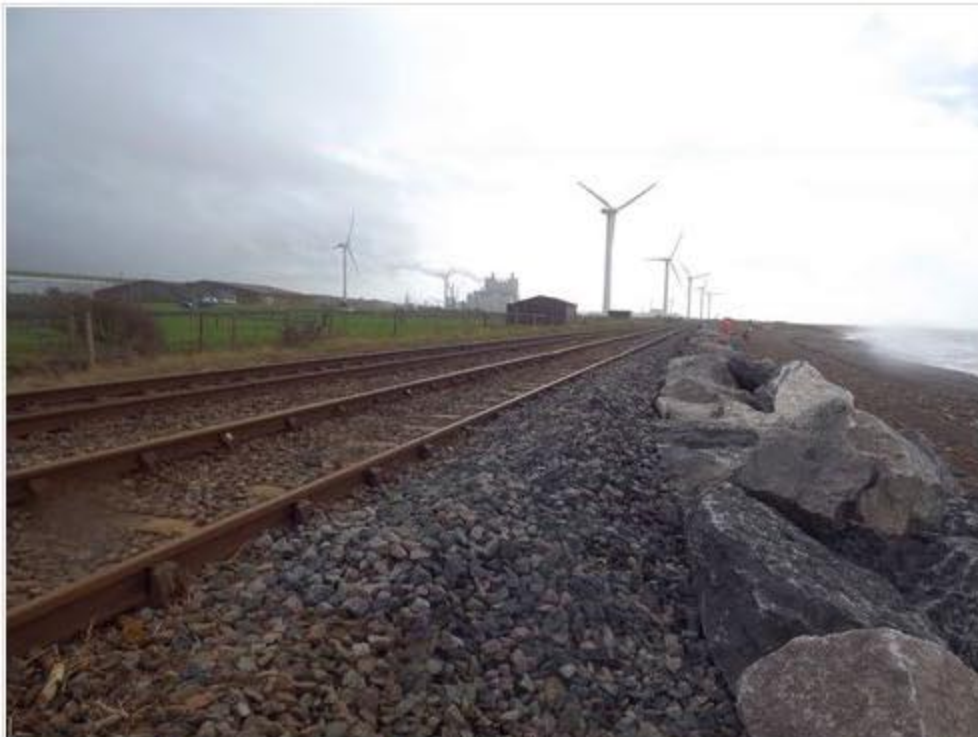
Temporary rock armour protects a length of railway having been recently reinstated after storms
